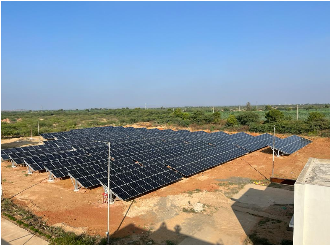
Ground Mounted Project
