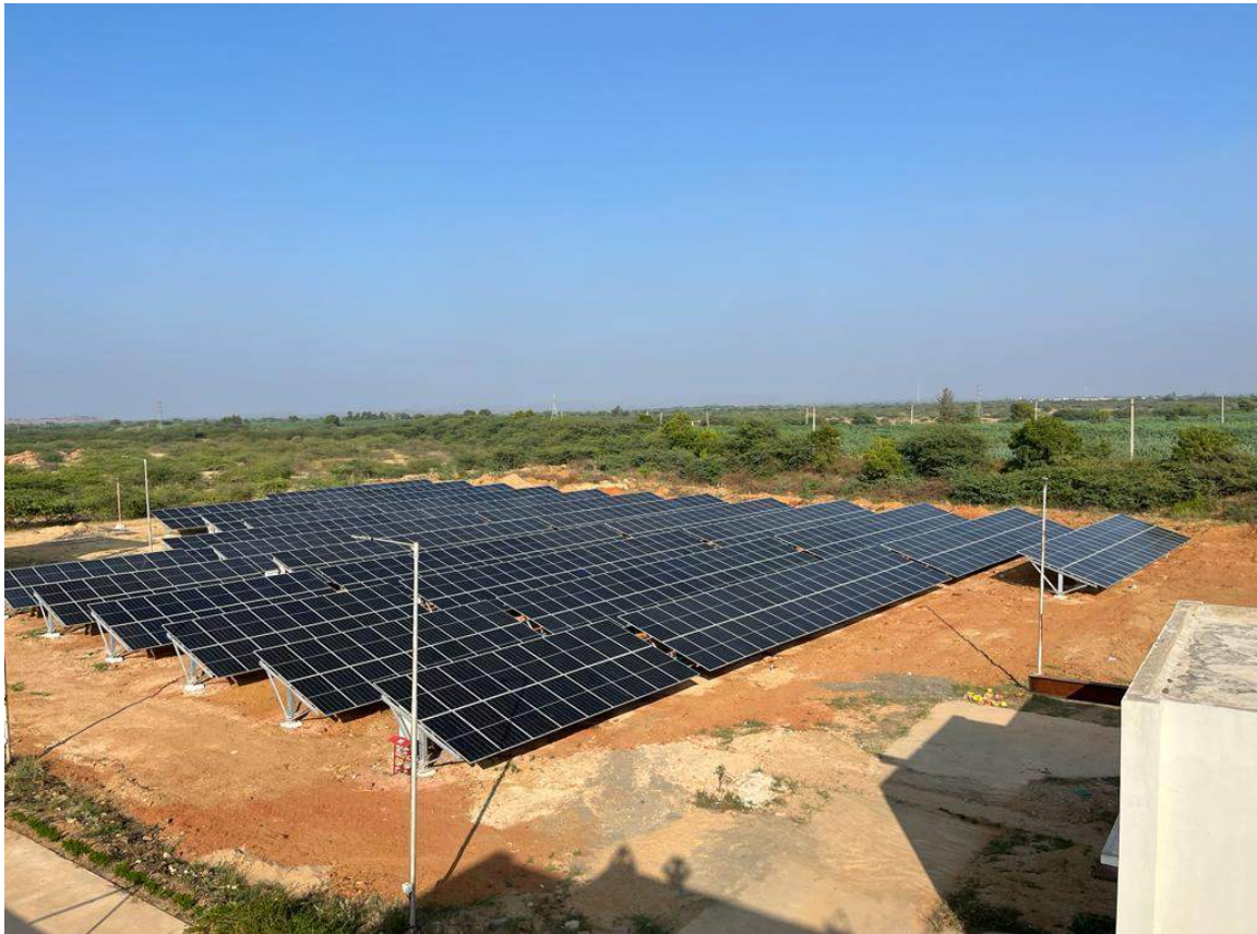
Ground Mounted Project
